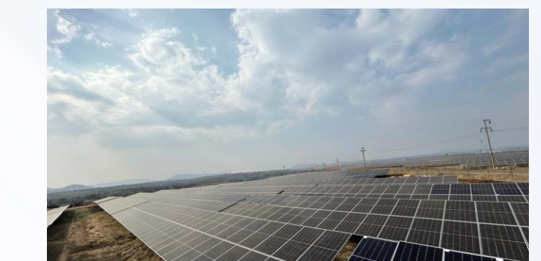
Solar Power Plant, Maharashtra (3.8 MW)
