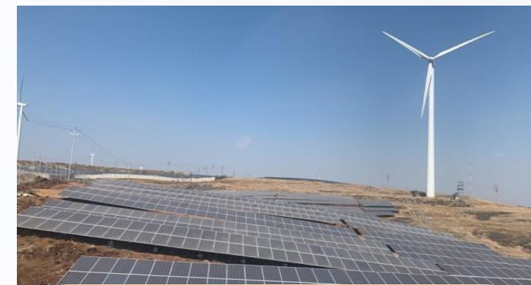
Solar Power Plant Ahmednagar, Maharashtra (5.2 MW)
